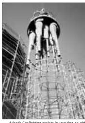
Atlantic Scaffolding assists in lowering an old regenerator head assembly into a temporary 'Jig stand' constructed from the EXCEL system.
