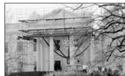
Atlantic Scaffolding erected a portico scaffold in front of the White House.
