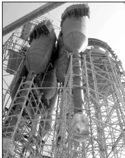
Atlantic Scaffolding's jig stand was used on an FCCU project, supporting the structure, as well as allowing for the human access needed to install the cyclones.
